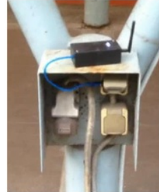
Fig. 16: Implemented transmitter module tested in a building area
